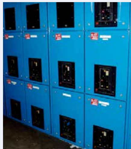
ACBs Merlin Gerin Selpact obsoletos
